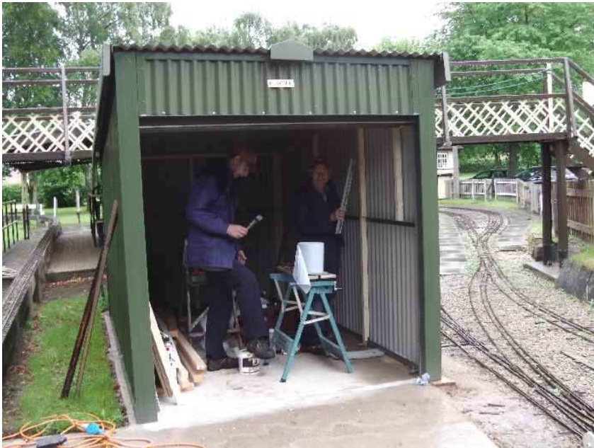
John and Peter at work in the new high level carriage shed
