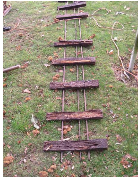
FOR ANYONE WITH ANY DOUBTS ABOUT REPLACING THE TRACK THIS SECTION SHOWS A DISASTER WAITING TO HAPPEN
